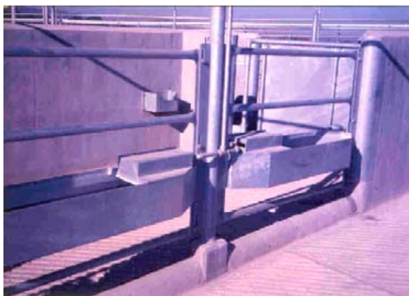
Fig. 22: Tubular rails and concrete walls for pen partition, non-slip concrete floor
