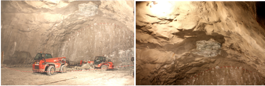
Figure 4. Zone of the incident near the tunnel face. Two equipment badly damaged (left). Detail of the rock detachment area at the tunnel roof (right).
