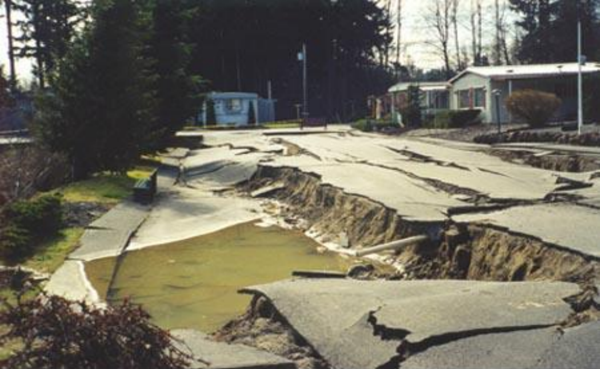
Tumwater, WA March 21, 2001 -- A road near the Tumwater Mobile Estates collapsed during the Nisqually Earthquake on Feb. 28.
