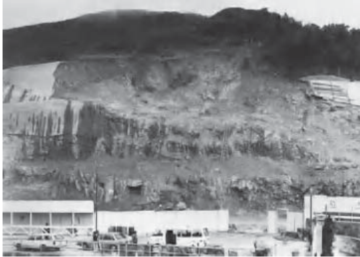
Figure B1-2.1 View of large rock slope failure in 1982, South Bay Close, Hong Kong.
