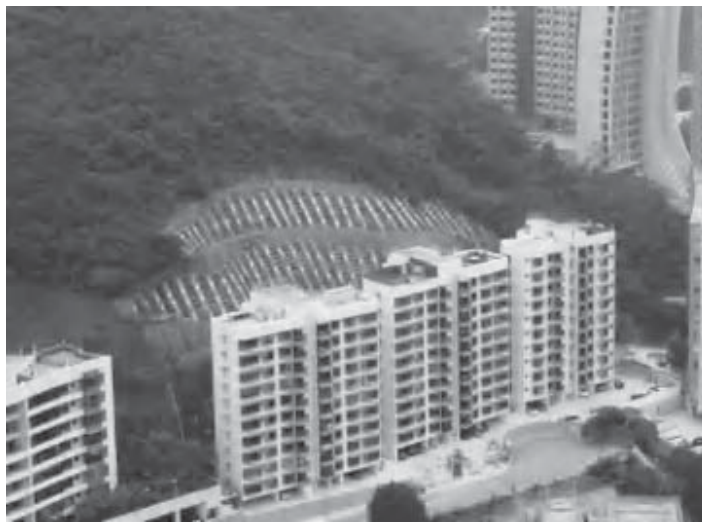
Figure B1-2.4 Slope in 2010 showing anchored concrete beams installed to prevent further failure in the trimmed-back slope above the apartment blocks.
