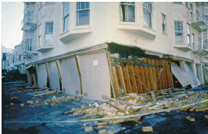
Figure 6.20 Earthquake damage Damage to buildings in the Marina district of San Francisco resulting from the 1989 M 7.1 earthquake. (John K. Nakata/ U.S. Geological Survey)
