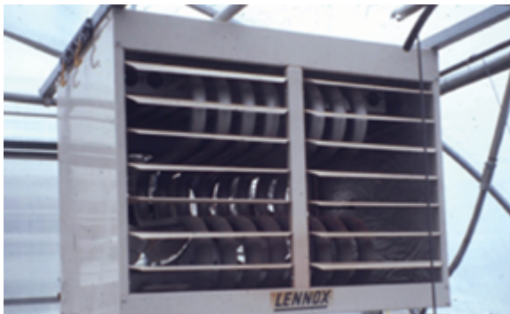
Unit heaters with HAF air circulation are a good choice for temporary heat.
