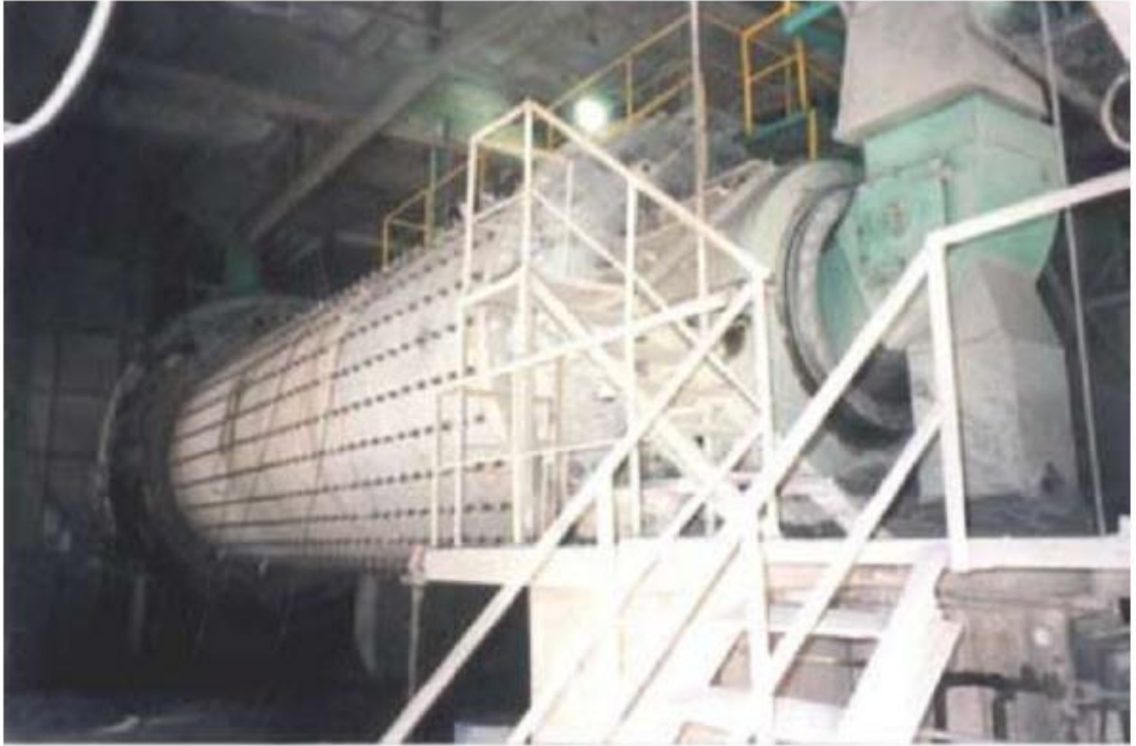
Photograph of a ball mill in a Cement Plant.
