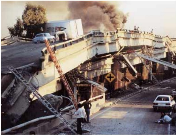
Figure 10-9 Surface waves cause a large proportion of earthquake damage. Collapse of Interstate Highway 880 during the 1989 Loma Prieta, California, earthquake. (Paul Scott/Sygma)
