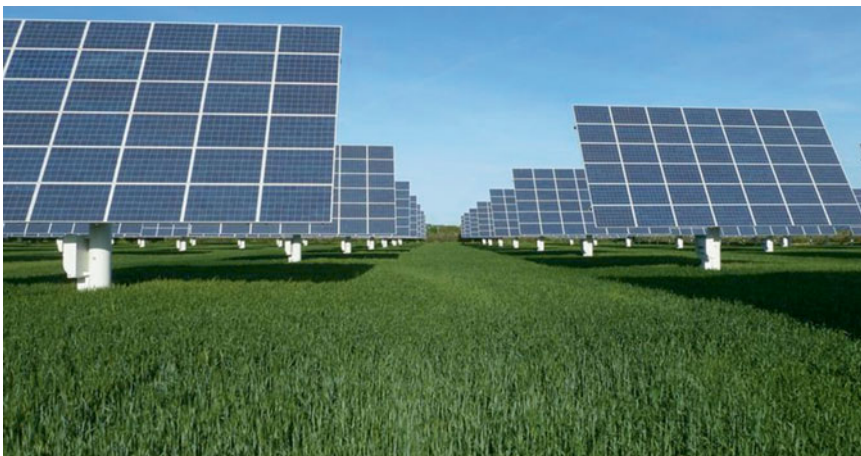
Fig. 12.13 Field filled with solar panels
