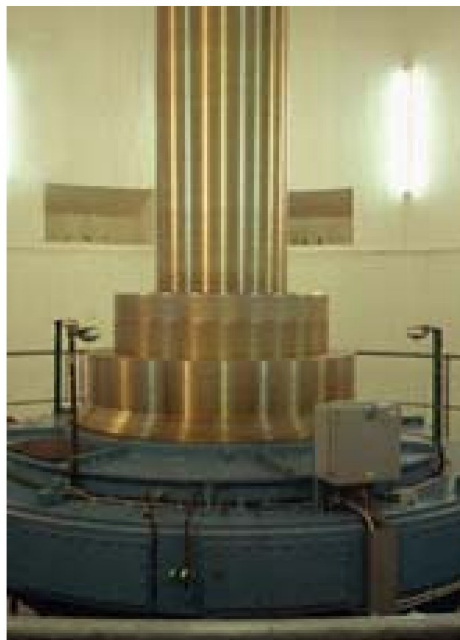
A big hydel generator. Governors are used to control the supply of working fluid (water in hydel generators).
