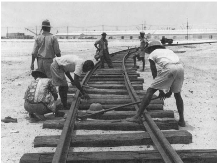
PHOTO 10.1 Workers repair track on Liberia's first railroad in 1950. This line connected the port of Morovia with the rich iron ore deposits in the Bomi hills. (Courtesy of the United Nations. Reprinted by permission.)
