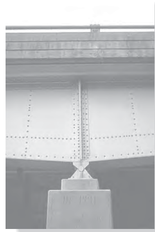
Typical pin used to support the steel girder of a railroad bridge.
