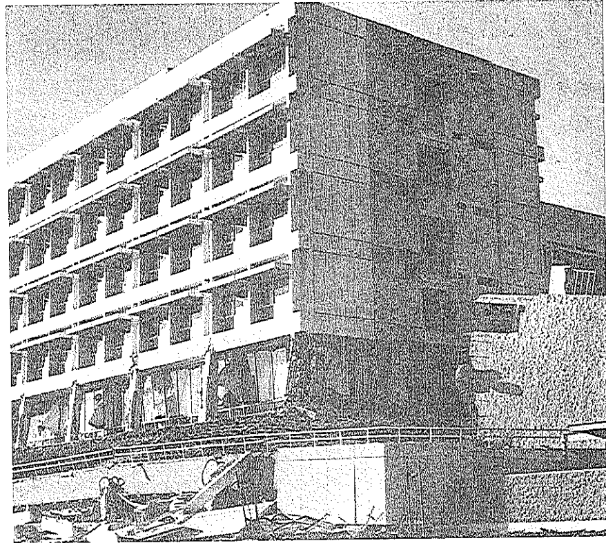
Figure 19.3.3 Olive View Hospital building. The shear walls in the upper four stories did not extend to the lower two stories. (From K. V. Steinbrugge Collection, courtesy of the Earthquake Engineering Research Center, University of California at Berkeley.)
