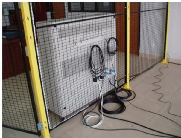
Fig. 1.11 Control Desk connected and ready for AC voltage measurement
