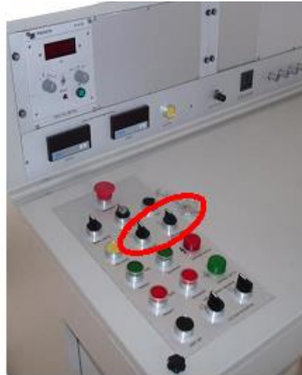
Fig 8.12 Sphere Gap Control Switches
