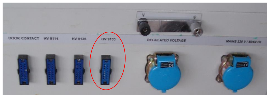
Fig 3.7 HV 9133 Sphere Gap Motor Control Input
