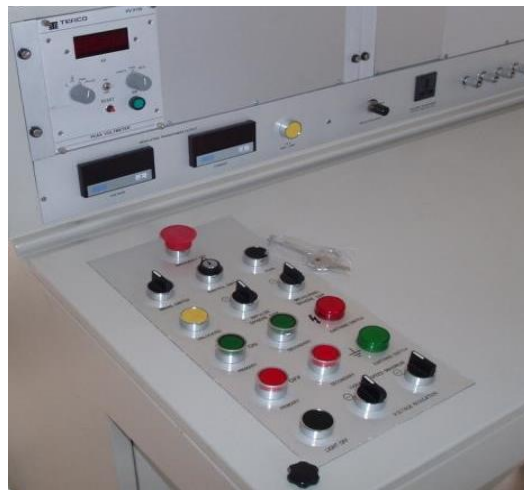
Fig. 3.8 Sphere Gap Adjustment Switches
