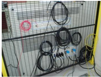
Fig 8.11 Control Desk Cables
