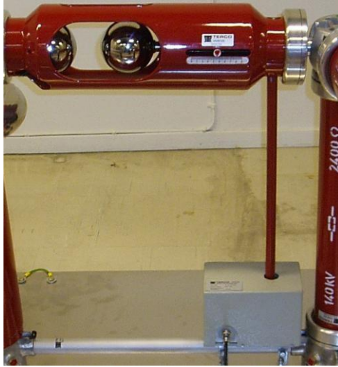
Fig 8.8 HV 9125 Sphere Gap and Drive
