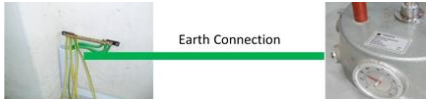
Fig. 3.6 Sphere gap Earth Connection point to bushbar
