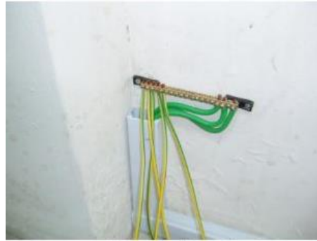
Fig. 1.4 (a) Earthing Bushbar
