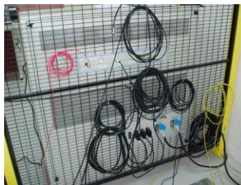
Fig 8.11 Control Desk Cables
