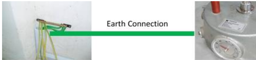
Fig. 3.6 Sphere gap Earth Connection point to bushbar
