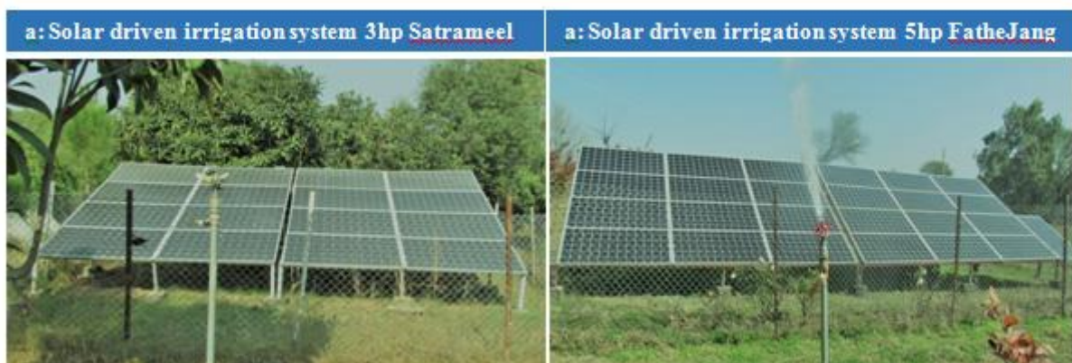
Figure 6: Solar powered pumping systems demonstrated at various sites
