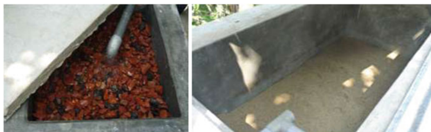
Fig. 9.4 River sand filter unit
