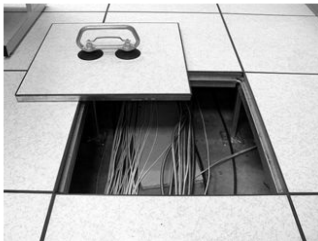
Picture 7: Removable tiles in a raised floor
