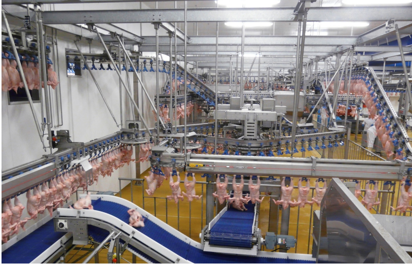
Figure 5.1.1.b Inside view of a modern poultry processing plant designed to handle 13,500 birds per hour. Courtesy of Marel.
