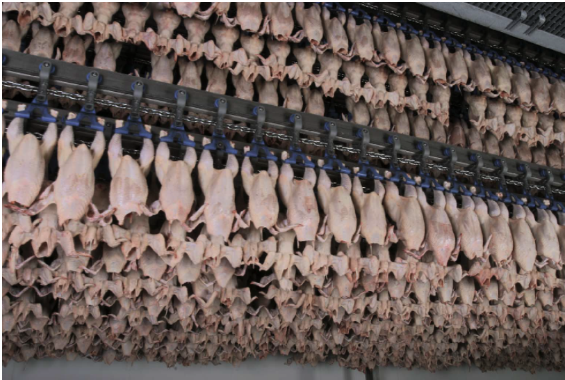
Figure 5.16.2 Air chilling system showing overall refrigeration area. Courtesy of Marel.
