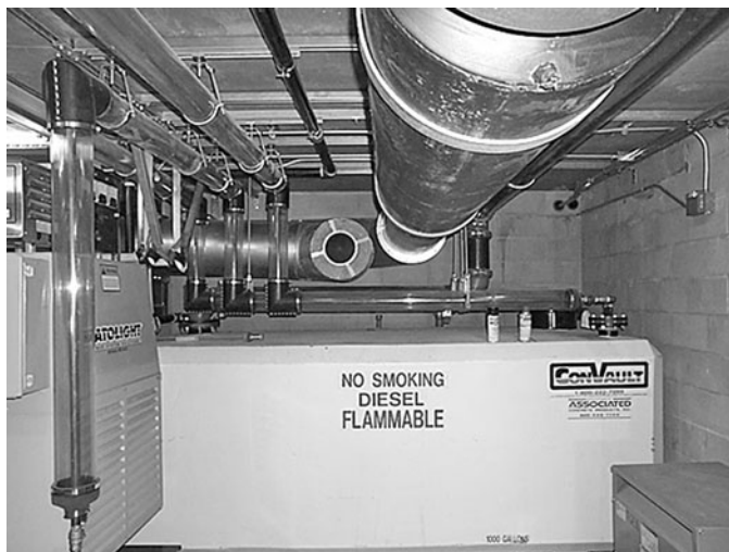
Figure 6.2 A 1,000-gallon tank to power the generators at GNAC, Inc.
