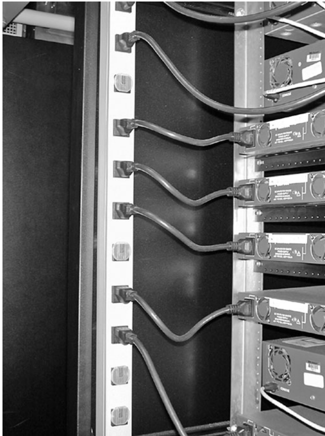
Figure 6.12 Vertical PDUs at GNAC, Inc., with short power cables are convenient and help to keep the wiring neat.
