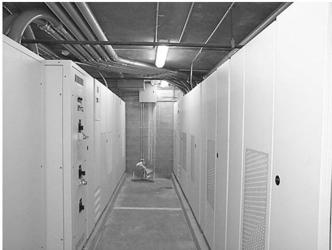
Figure 6.1 A modular UPS at GNAC, Inc.
