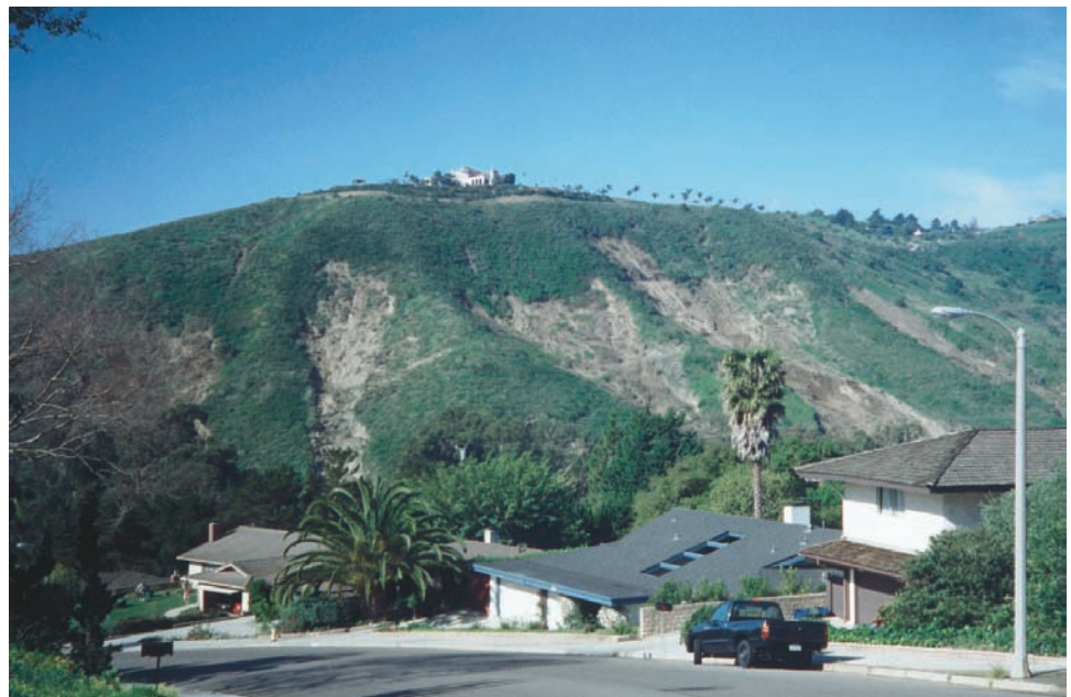
Figure 1.11 Urban development The presence of a landslide on this slope suggests that the slope is not stable and further movement may occur in the future. This is a “red flag” for future development in the area. (Edward A. Keller)
