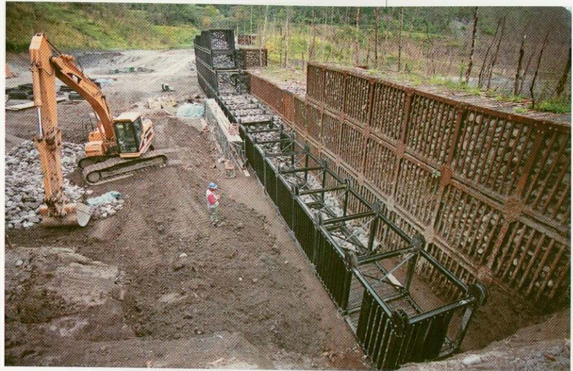
▲ Fig. 13.27. Enlargement of sabo dam by rock fill on the flanks of Usu volcano near Toya following the eruption in 2000
