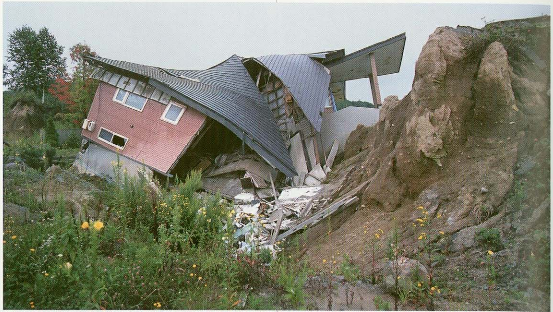
► Fig. 13.19. Collapsed house next to fault scarp with 10 m displacement, the result of domal uplift during the 2000 eruption of Usu volcano (Hokkaido, Japan)
