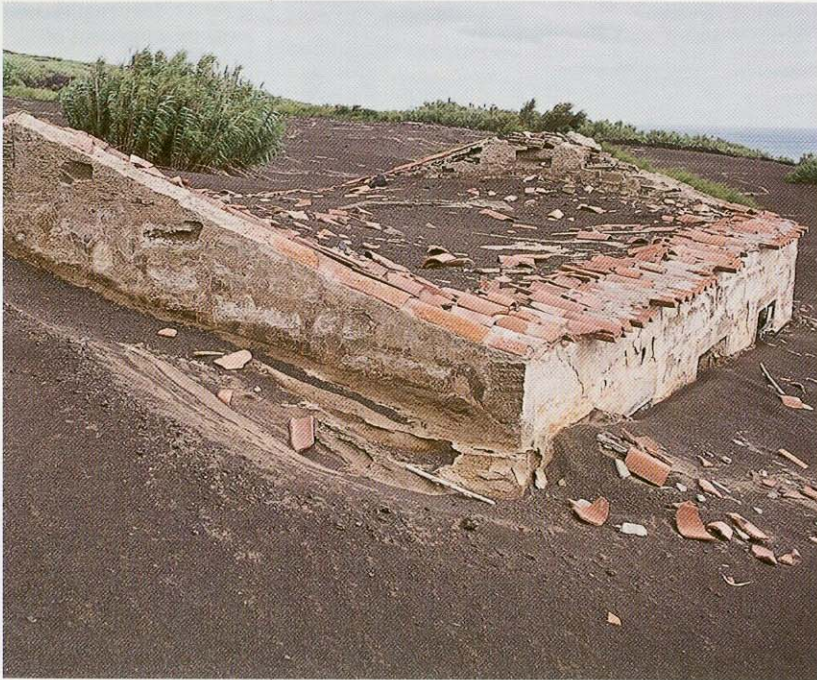
◀ Fig. 13.11. House buried by ashes generated during a phreatomagmatic eruption of Capelinhos volcano off the coast of Fayal (Azores). See also Fig. 12.2
