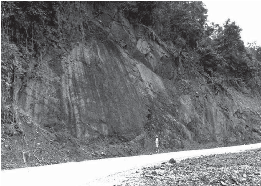
FIGURE 1.101 The face of the major joint surface in siltstone is stable but the overhanging blocks will fail along the same surface unless removed or retained (Sidikalang, Sumatra).
