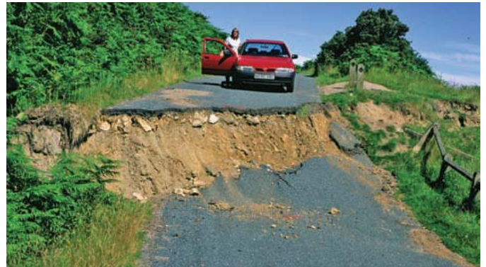
Head scar of a rotational slide breaks a road in Yorkshire.
