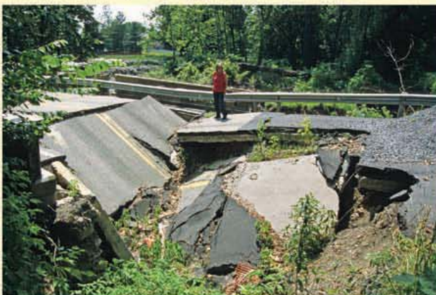
Subsidence sinkhole near deep limestone quarry, Pennsylvania.
