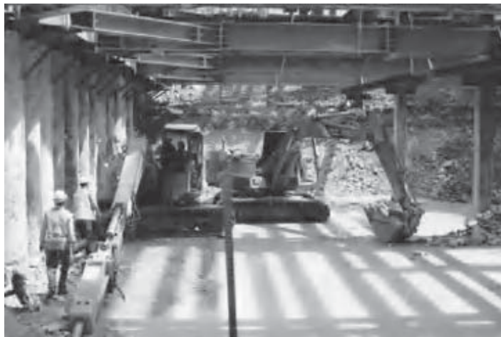
Figure 6.2 Temporary works for an underground station construction in Singapore. Piles to the left were excavated by a large-diameter drilling rig and then concreted. As excavation has proceeded, the piles have been anchored back into the ground and strutted using systems of waling beams (horizontal, along the face of the piles) and struts, supported where necessary by additional king posts.
