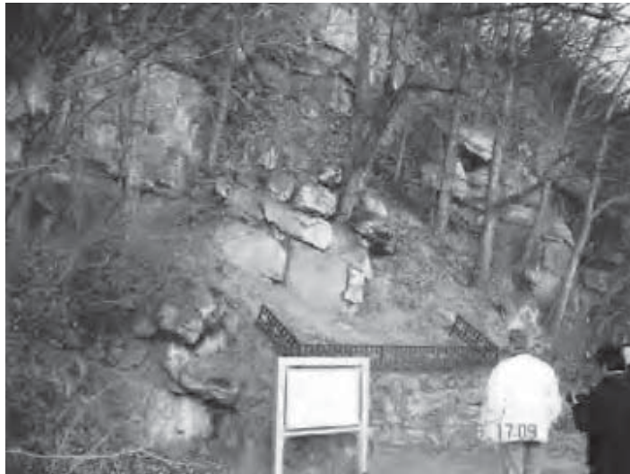
Figure B6-4.1 Petroglyphs at Anhwa-ri, Goryeong, Korea. Rock slope above petroglyphs (with small protective fence) shows signs of vegetation wedging, with loose blocks resting against trees.
