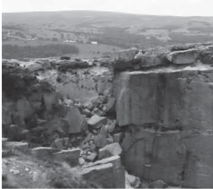
Figure B6-4.2 Unexpected rock failure in Cow and Calf Quarry, Ilkley, West Yorkshire, UK.
