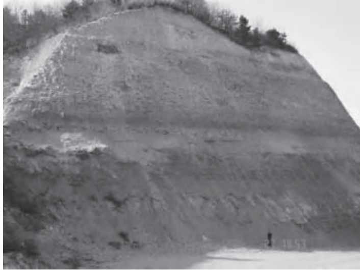
Figure B6-5.1 View of large cut slope in Eocene mudstone near Po Chang Korea.
