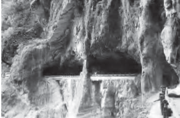
Figure B6-4.3 Road cut through limestone with very little engineering support or protective measures, Tailuko Gorge, Taiwan.
