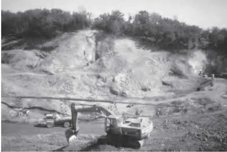
Figure B5-1.1 View of left abutment of Queen's Valley Dam, Jersey, UK, under construction.
