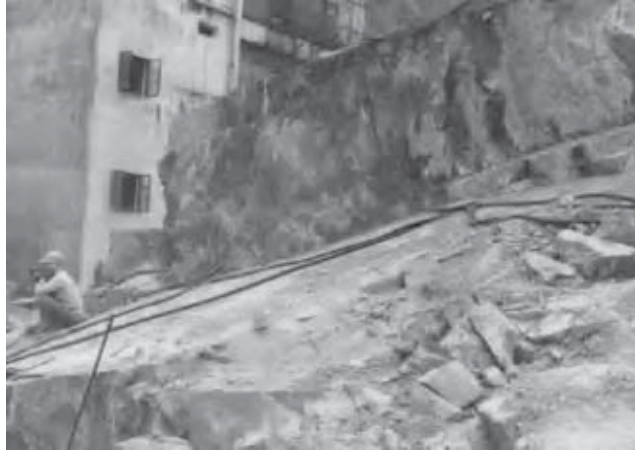
Figure B5-2.1 Failure plane with debris cleared off.
