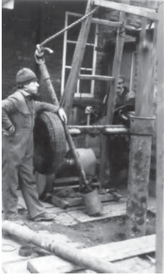
Figure 4.22 Shell and auger rig in action, Leicester, UK. Casing, used to support the hole, is standing out of ground and a shell is being dropped down hole to excavate further. In the foreground is a U100 sampling tube attached to a down-hole hammer, ready for placing down hole and taking a sample once the hole has been advanced to the required depth. Leaning against the wheel is one of the drillers and also a trip hammer for SPT testing – also awaiting use at appropriate depths and changes in strata.
