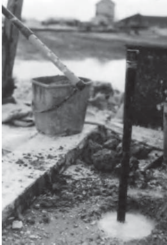
Figure 4.40 Standpipe piezometer tip about to be placed in borehole. Another has already been installed at a deeper level. It is not very good practice to install more than one piezometer in a borehole, because of potential leakage between the different horizons being monitored, but can work providing great care is taken in installation. Portsmouth dry dock, UK.
