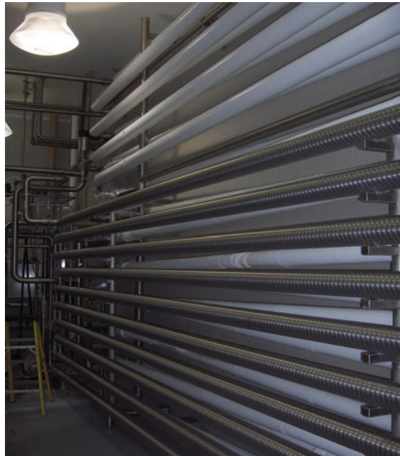
Figure 19.5 Liquid egg products are pasteurized using tubular-type high-temperature-short-time (HTST) systems. Courtesy of Dr Vincent Guyonnet of Burnbrae Farm Ltd., Canada.
