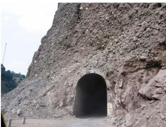
Fig. 4 Destruction of the tunnel opening on the road located in the south of Muzaffarabad
