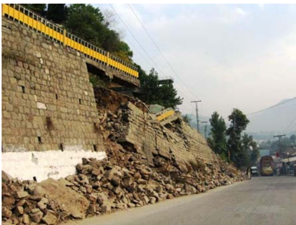
Fig. 8 Muzaffarabad: the retaining wall collapse due to Balakot earthquake mainshock on 8 Oct. 2005
