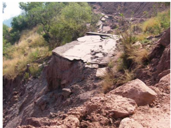
Fig. 2 Islamabad–Muzaffarabad road destroyed by Balakot earthquake on 8 Oct. 2005
