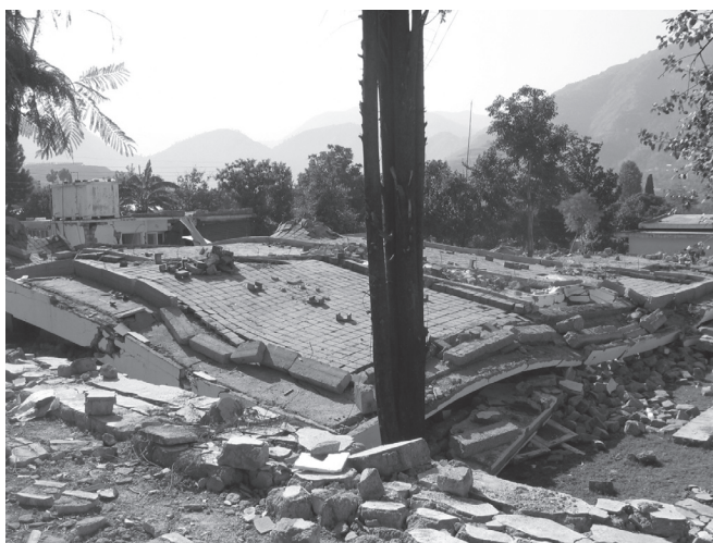
▲ Figure 24. Heavy roof (Muz).
