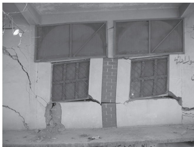
▲ Figure 26. Shear cracks (Muz).
