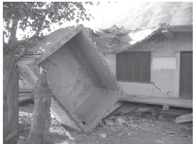
▲ Figure 21. Large water tanks at roof (Muz).
