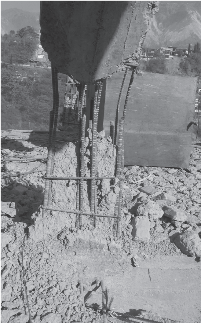
▲ Figure 14. Lateral confinement of concrete (Blk).
