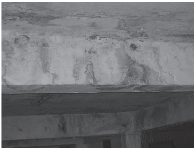
▲ Figure 23. Seepage and maintenance problem (Isb).
